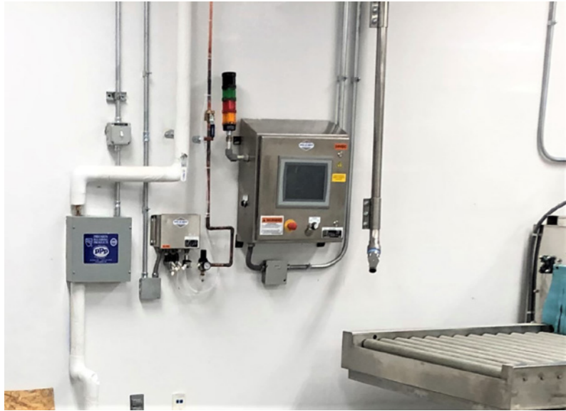
NEMA 4X control panel for washdown environment with water-shed design.
